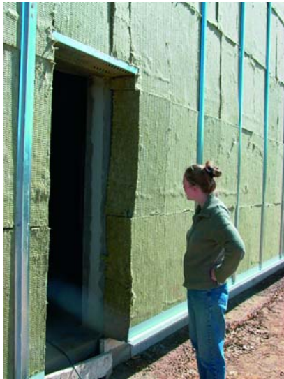
Figure 2. Erecting the walls in June 2003. The climate is stabilized by solid walls of 240 mm open-pored concrete. Note the 250 mm isolation on the outside of the wall
